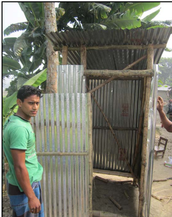
Portable toilet frame has been built and later will be placed near the houses...
