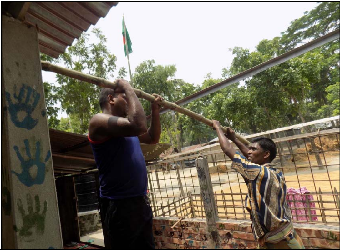
Last April storm damaged the school, we repaired...
